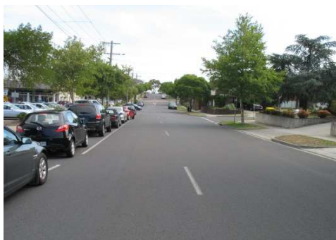
Faded Line Marking - Grant Olsen Avenue
