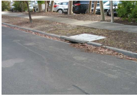
Blocked Pit – Derreck Avenue -
