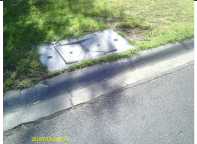
Damaged Pit Insert
