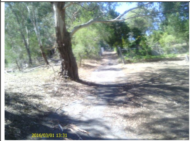
Tree Root damage
