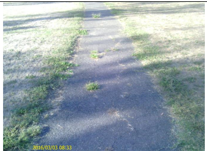
Footpath Weed Infiltration
