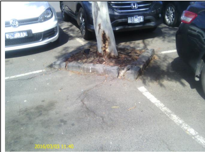
Car park Tree Root damage
