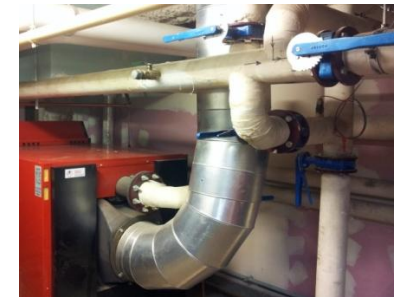
Civic Offices ductwork – leaks tend to occur at every join in the rigid ductwork
