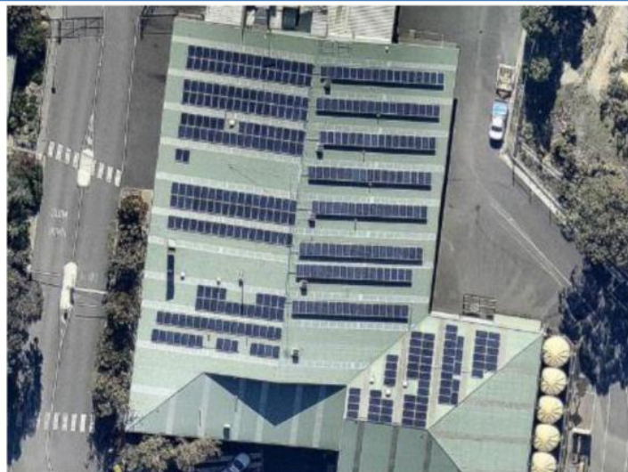
Depot rooftop with completed 99kW Solar PV array
