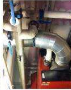
Civic Offices ductwork – leaks tend to occur at every join in the rigid ductwork
