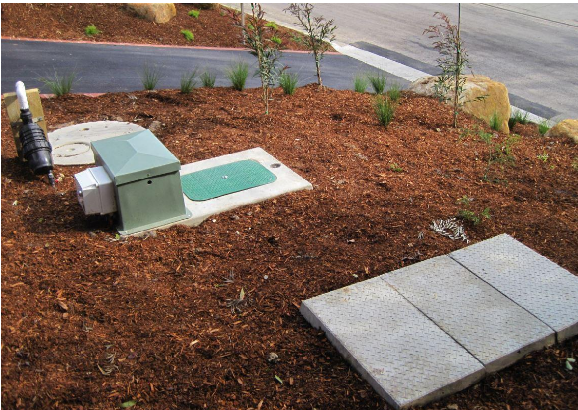
Figure 3: Treatment Plant with sub-surface irrigation
