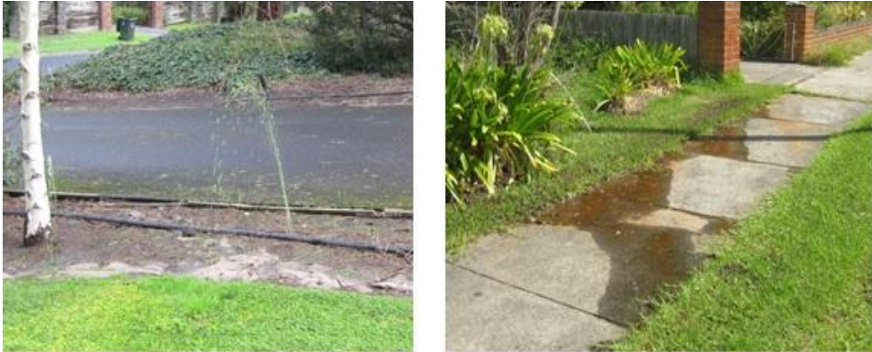
Figure 7: Burst dripper line and septic effluent flowing over footpath
