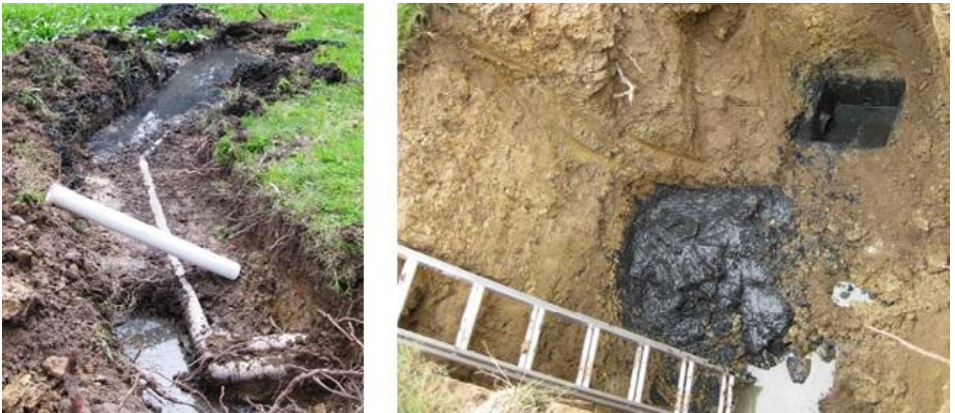
Figure 8: Flooded irrigation field and a deeply buried distribution pit (legacy system)
