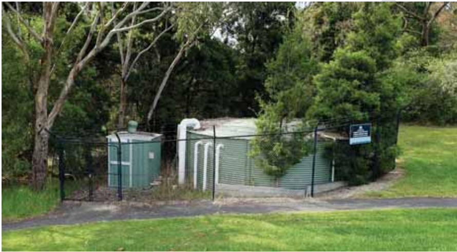
Figure 5: Stormwater harvesting plant at Domeney Reserve, Park Orchards
