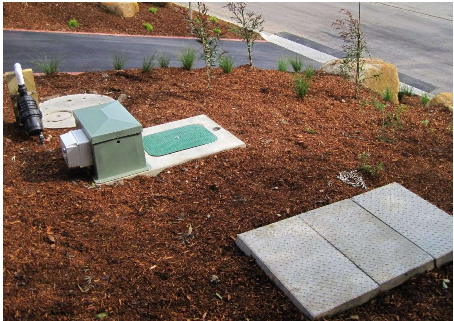
Figure 2: Treatment Plant with sub-surface irrigation
