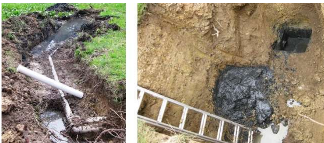
Figure 11: Flooded irrigation field and a deeply buried distribution pit (legacy system)
